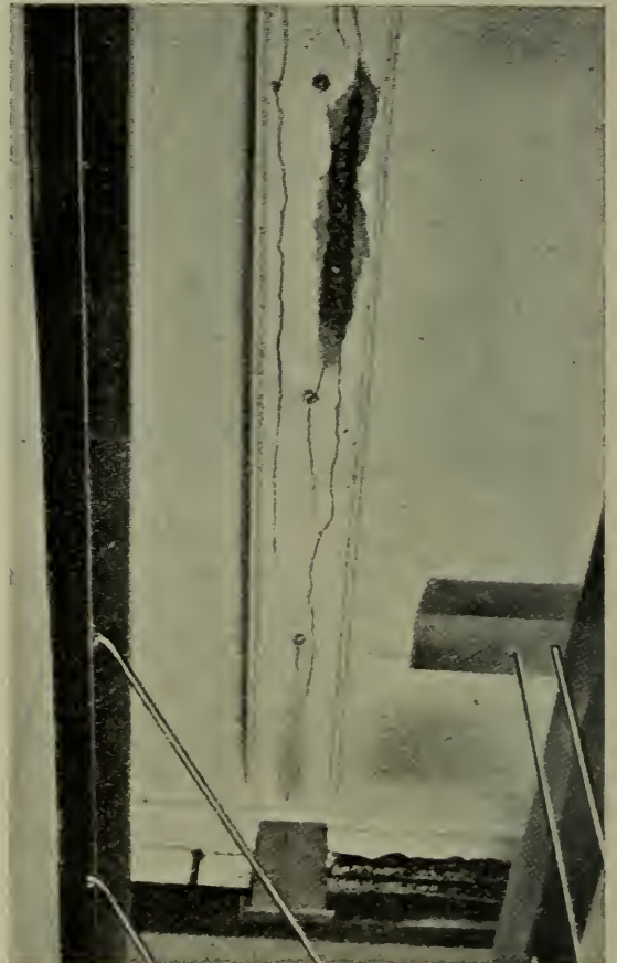
FIG. 8. ELECTROLYTIC CORROSION OF STEEL REINFORCEMENT: CRACKS IN LOWER PART OF GIRDER.
